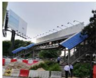
Final connection of the proposed bridge to the existing bridge that connects to the Damansara Intan.
